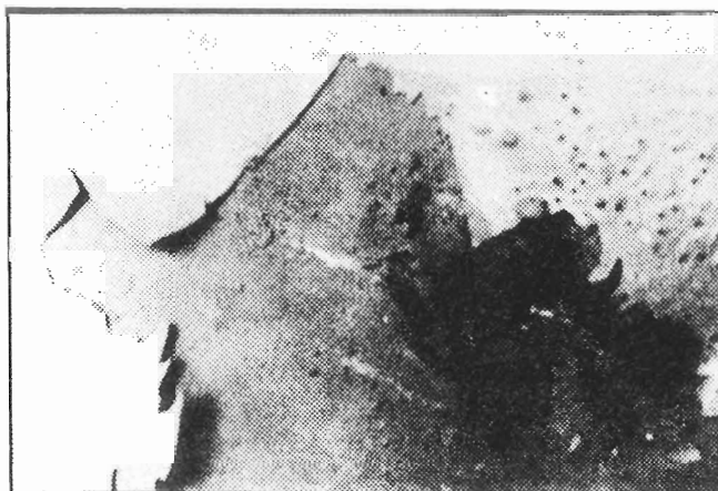
Lifting off of a coating caused by application on a moist surface
